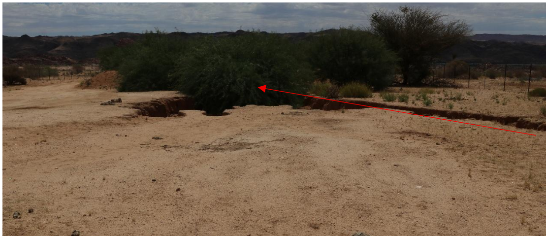
Figure 8: One of the affected drainage lines is situated within the existing sewage disposal pit, resulting in obstruction of flow and erosion. This can be avoided by diverting flow around the perimeter of the proposed WWTW.
