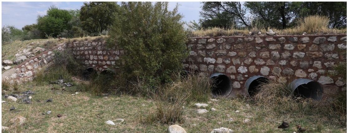
Figure 10: The existing road and culvert crossings also act as barriers to unimpeded flow and in several instances, culverts have become blocked or obstructed, which will further affect the natural flow of these watercourses.
