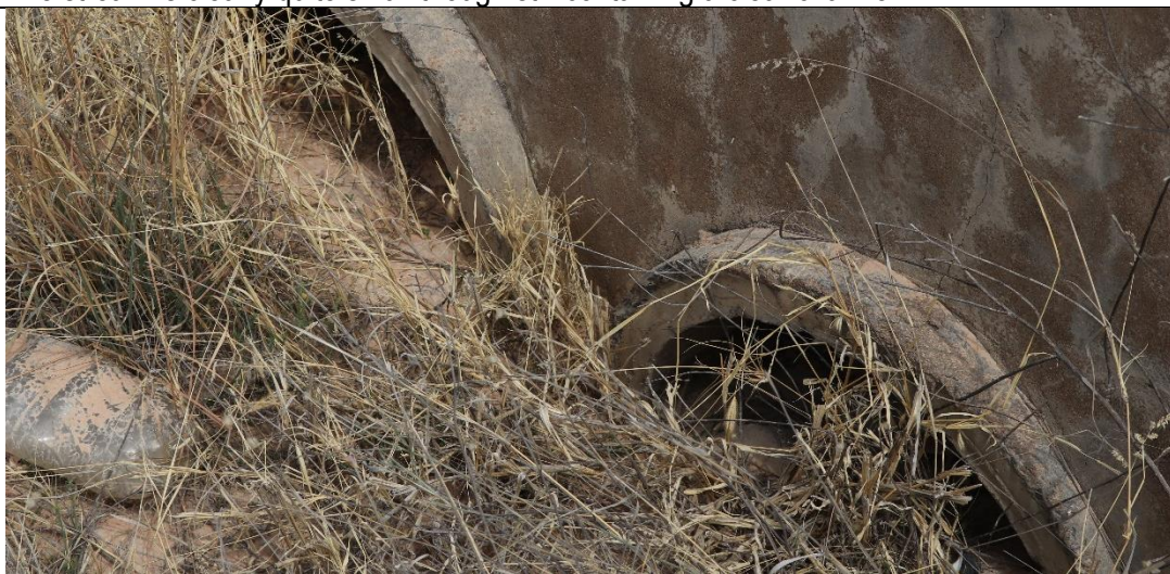
The stream is affected by several impacts and sedimentation is clearly problematic. Note how culverts have become almost completely blocked by sediment accumulation.
