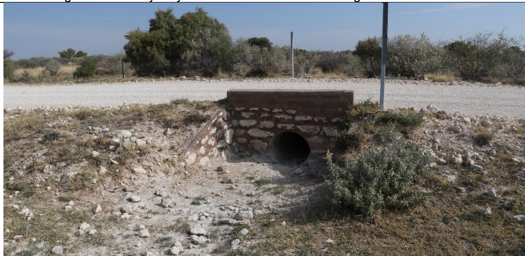
The small culvert will still facilitate flow, but will most likely also cause some constriction of flow.
