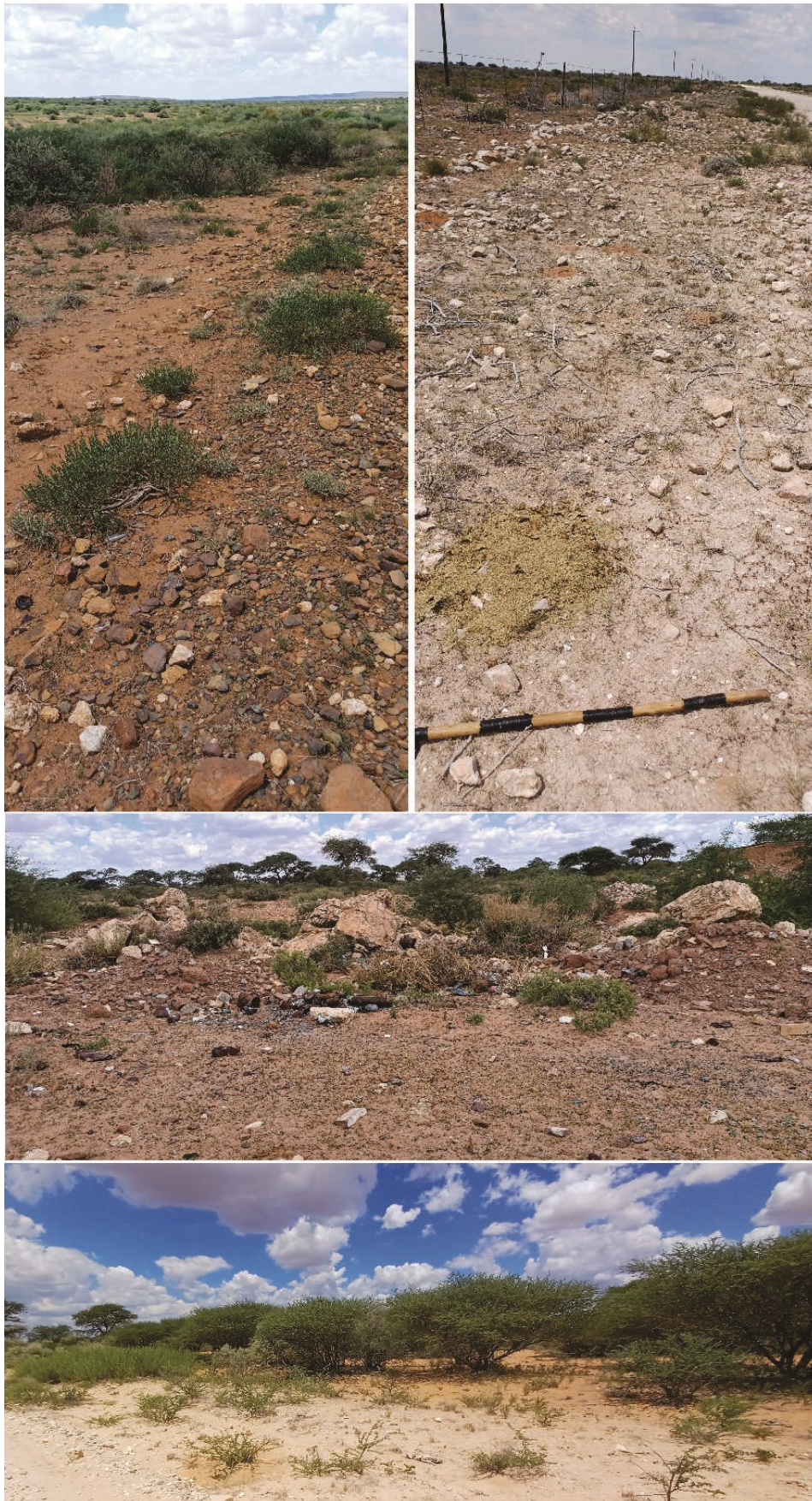
Figure 7. The road reserves are capped by severely degraded surface limestone rubble and residual soils (windblown sand) resulting from the construction of the existing road
